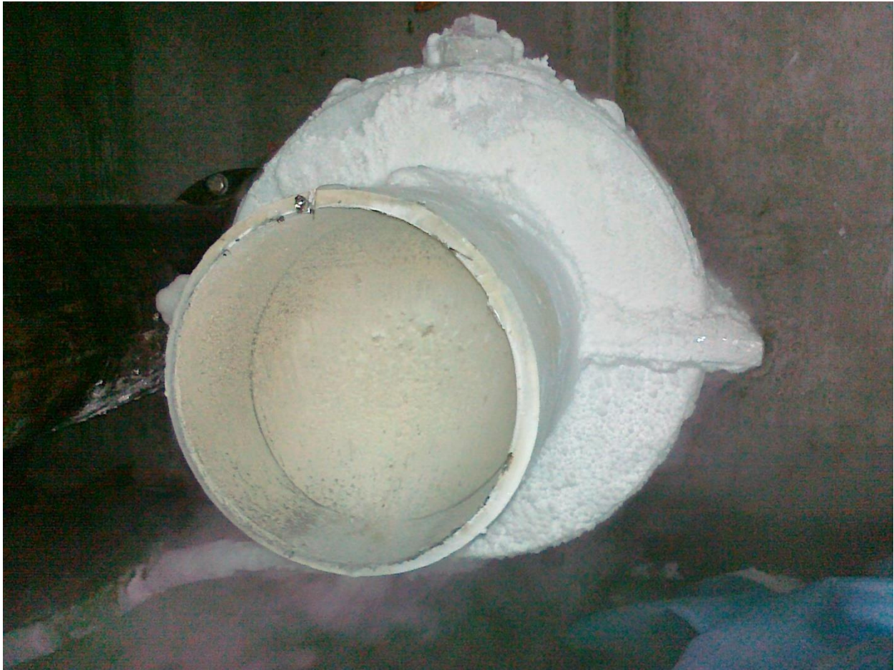
After the freeze, the pipe segment is cut, can see the ice plug
